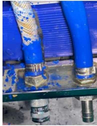
Figure 2: Degraded vs. intact blue colored hose
