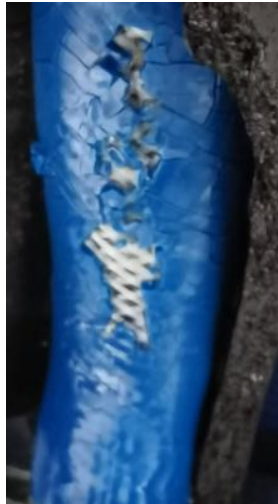
Figure 1: Degraded drain hose
